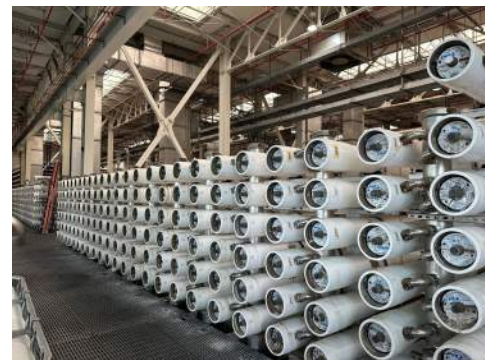
Figure 6: AWP facility in California: view of the reverse osmosis (RO) system. September, 2024. Credit: Roberta Santos
