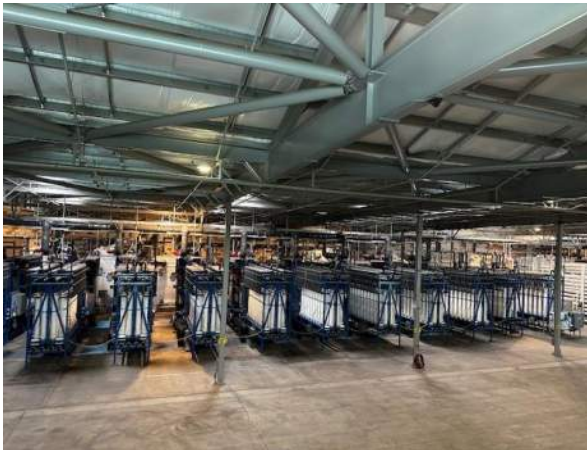
Figure 1: Site visit to an AWP facility in California view of the RO system. September, 2024. Credit: Roberta Santos
