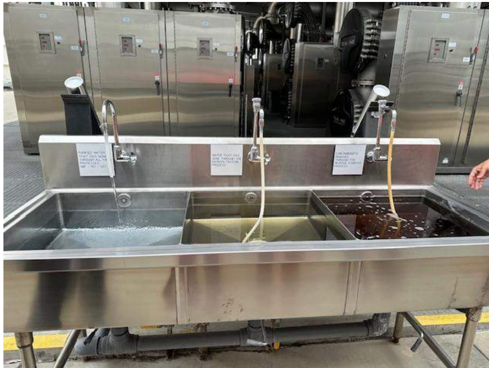
Figure 12: Water station at a AWP California treatment facility illustrates the process from untreated water (right) to AWP-treated drinking water (left). September 2024. Credit: Roberta Santos
