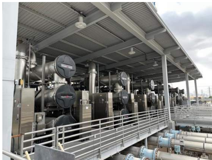
Figure 9: AWP facility in California: view of the ultraviolet (UV) disinfection system. September 2024. Credit: Roberta Santos
