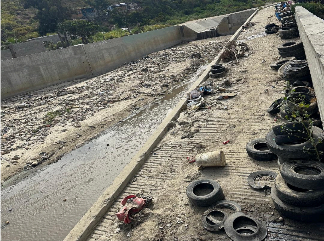
Image Eleven: A catch basin filled with tires and sediment.
