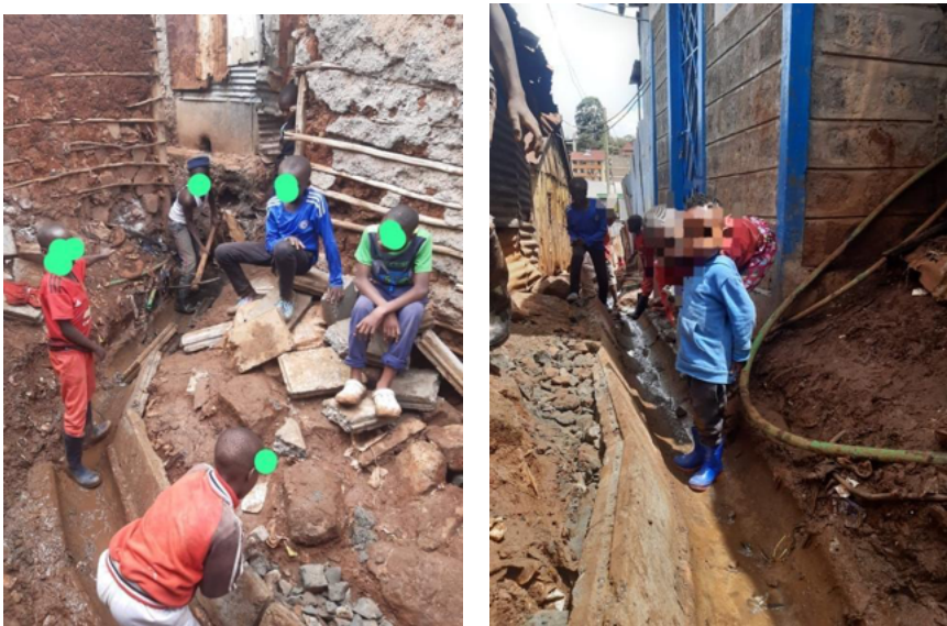
Figure 8 Before, during-construction, and after-construction images of the drainage channel. A community-driven initiative by the youth and children
