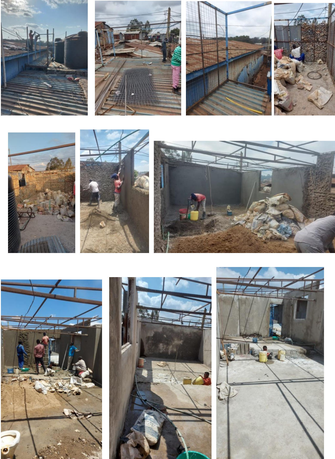
Figure 9 The construction process of a new community hall that serves as a space for residents to gather for games and watch football matches. The hall is made entirely from recycled C&D waste.
